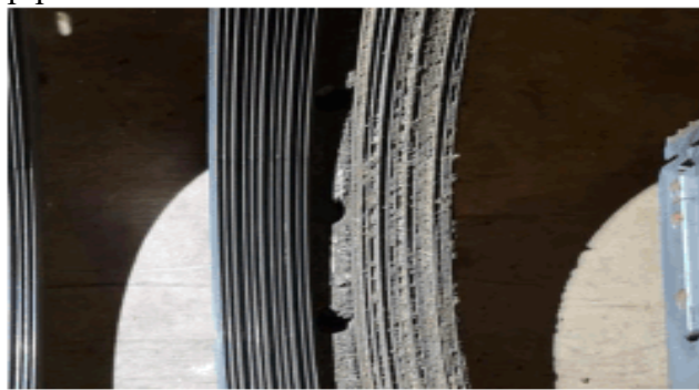
Figure 5. Oil sludge on the intermediate pressure rear shaft steam sealing ring
