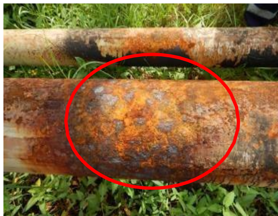
Gambar 2 korosi Intergranular Corrosion
