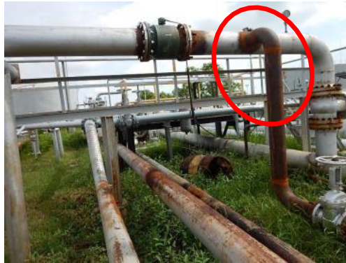
Gambar 3 korosi Galvanik Corrosion
